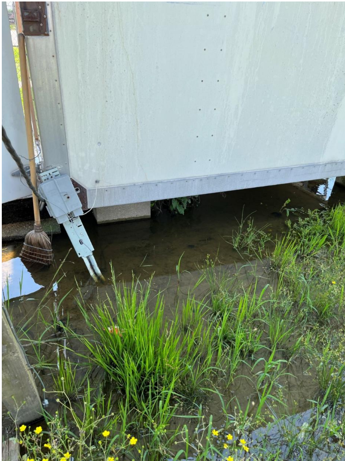
Figure B3: Current Marion Site, Exterior; Flooded conditions day after rain at side of structure
