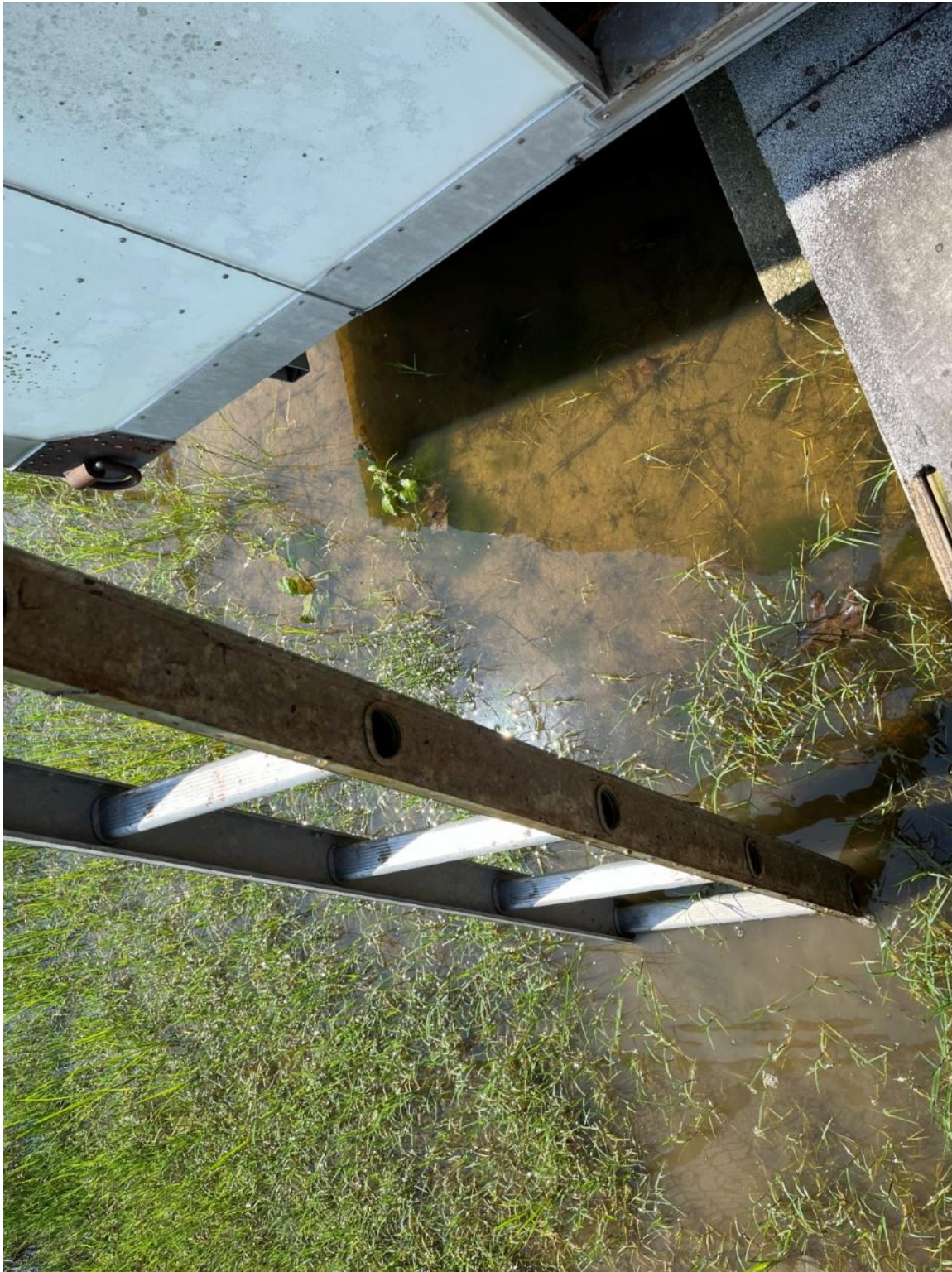
Figure B2: Current Marion Site, Exterior; Flooded conditions day after rain at entrance to structure
