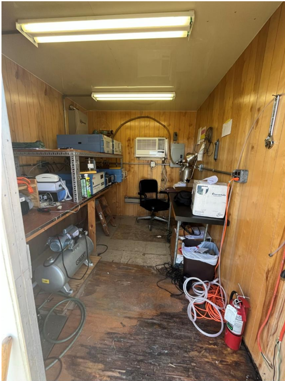
Figure B6: Current Marion Site, Interior; Floor, wall, roof damage from flooding conditions
