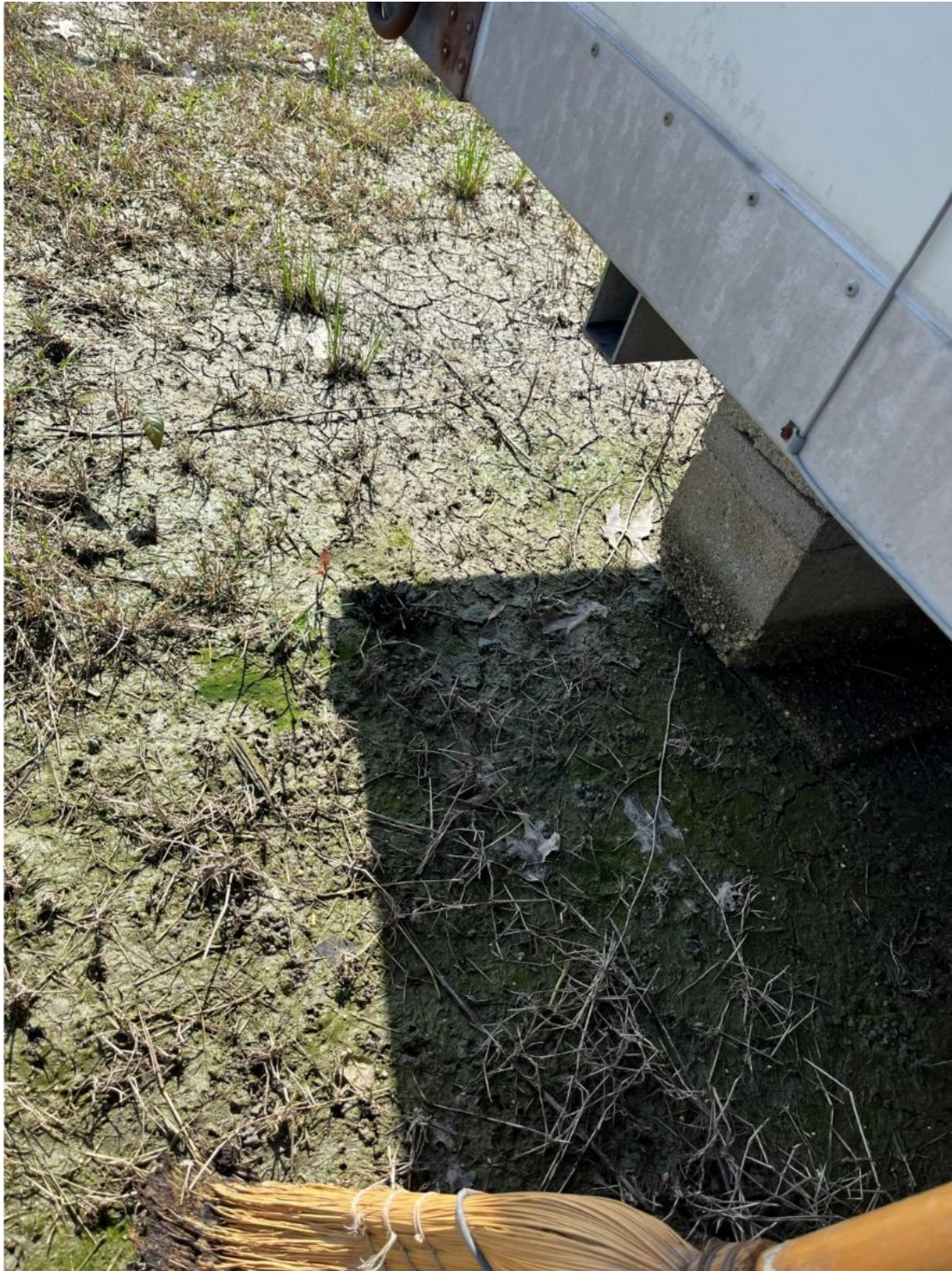
Figure B4: Current Marion Site, Exterior; Muddy conditions week after showing waterlines on structure and erosion damage to supporting feet
