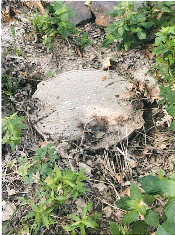
MH 12242 - Before repair
