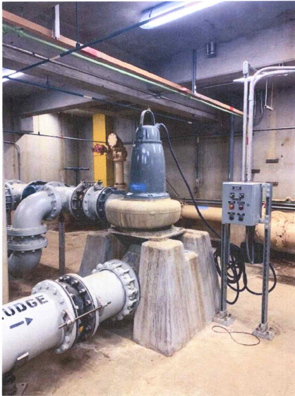
East Sludge Tank Pump Installed
