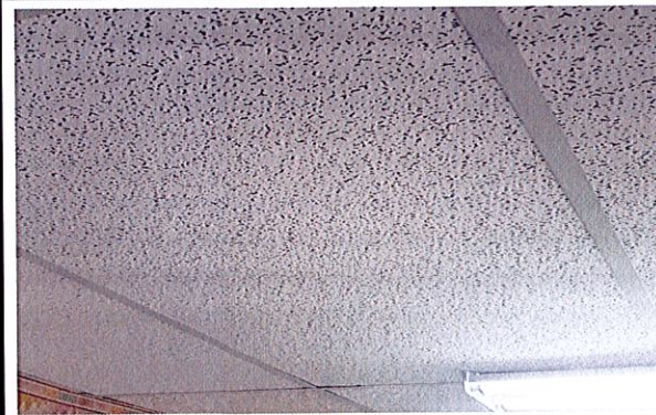
4771-24-47 & 48 2x4 Lay-in Ceiling Tile (Type III)
