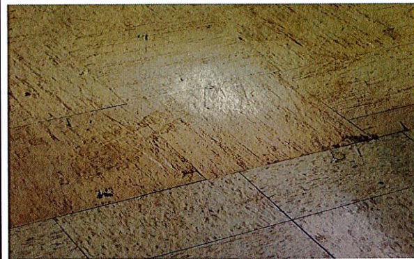
4771-19-37 & 38: Dark Tan 12x12 FT / Mastic - 5% Chrysotile
