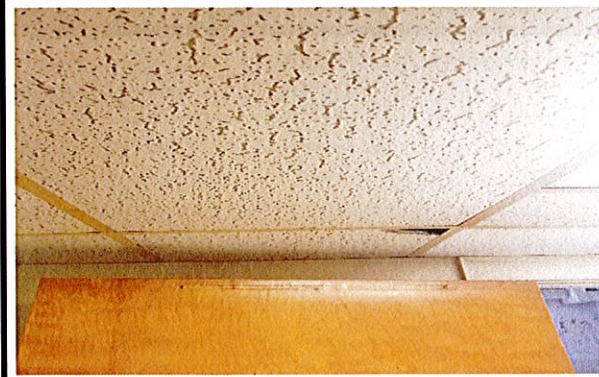
4772-04-07 & 08: 2x4 Lay-in Ceiling Tile (Type III)
