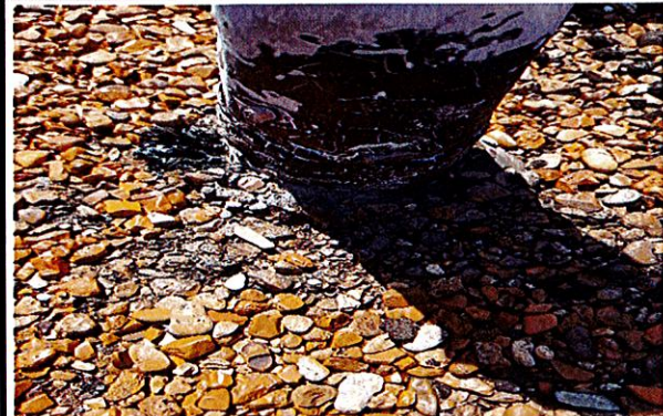
477R-02-02: Lower Roof - Penetration Mastic - 20% Chrysotile
