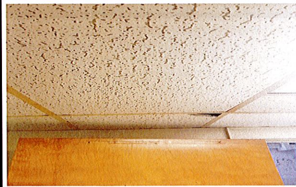
4772-04-07 & 08: 2x4 Lay-in Ceiling Tile (Type III)
